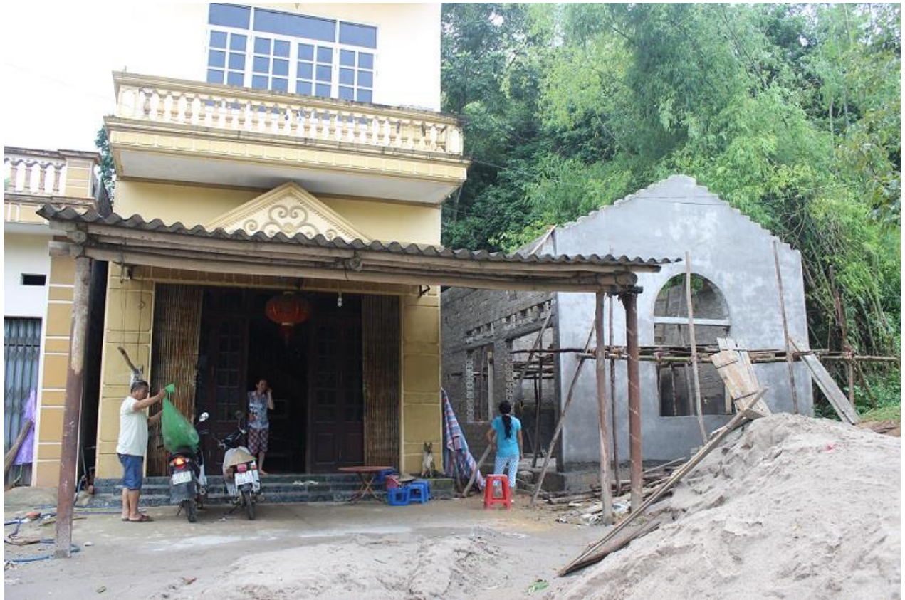
A new guesthouse is being built in Khun Phang village, Quang Lang commune
